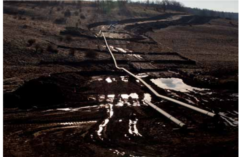
Gas pipeline near East Smithfield, PA.
