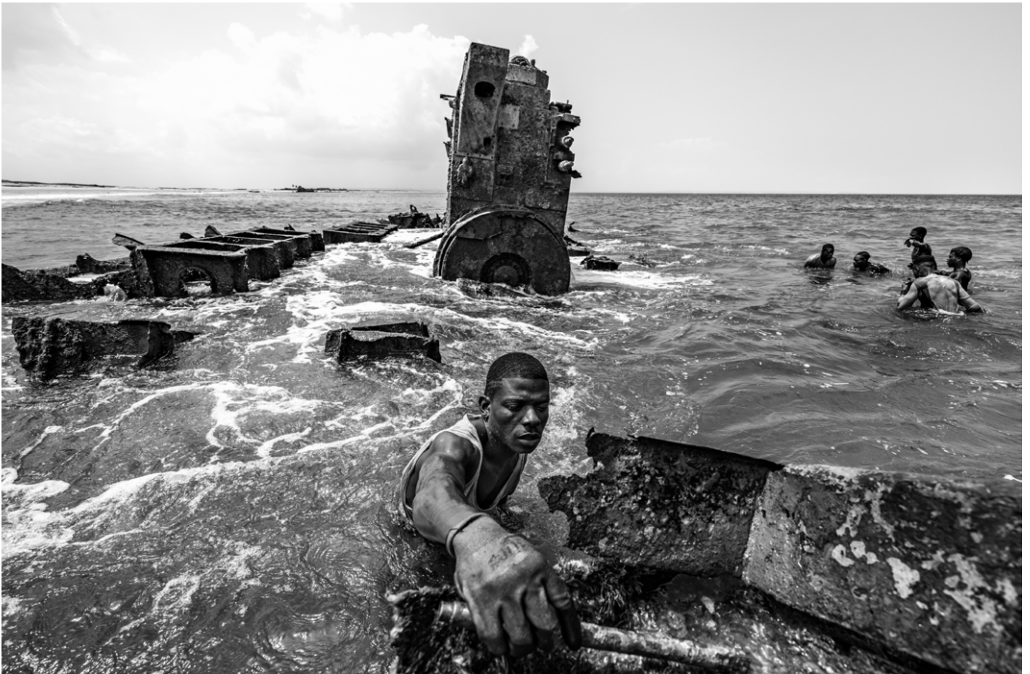
The danger of lifting and moving heavy pieces of sharp and corroded iron in water that is deep and constantly shifting is a significant part of an average workday.
